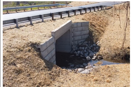
In conjunction with US Bridge, County Forces replaced our Greenfield 22 Bridge on Camp Ground Road. (pictured above).
